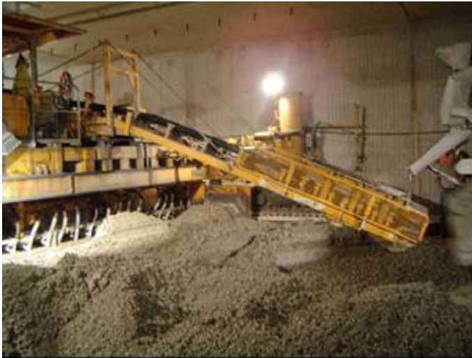
Figure 5. Two layer concrete pavement, wet-in-wet: supply of concrete of the upper layer over the first slipform paver
