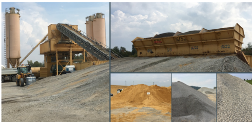
Figure 5. A concrete batching plant with different stockpiles of aggregates
