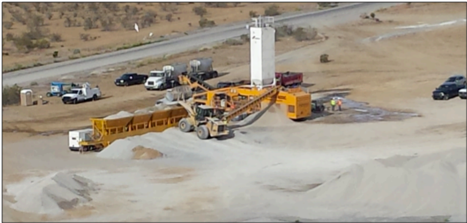
Figure 10. Pugmill Mixing Plant
