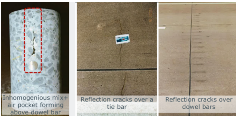
Figure 3. Problems on single layer JPCP by the use of an automatic DBI
