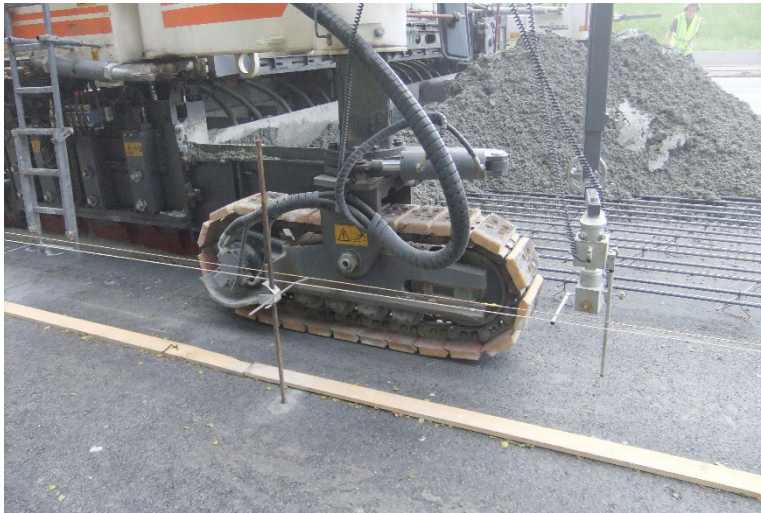
Figure 2. Rolling path of the tracks on an asphalt sandwich layer.
