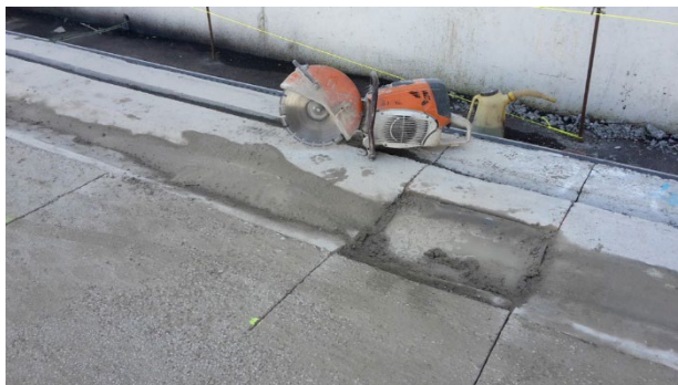
Figure 6. Cutting of the active crack control immediately after washing of the surface each
