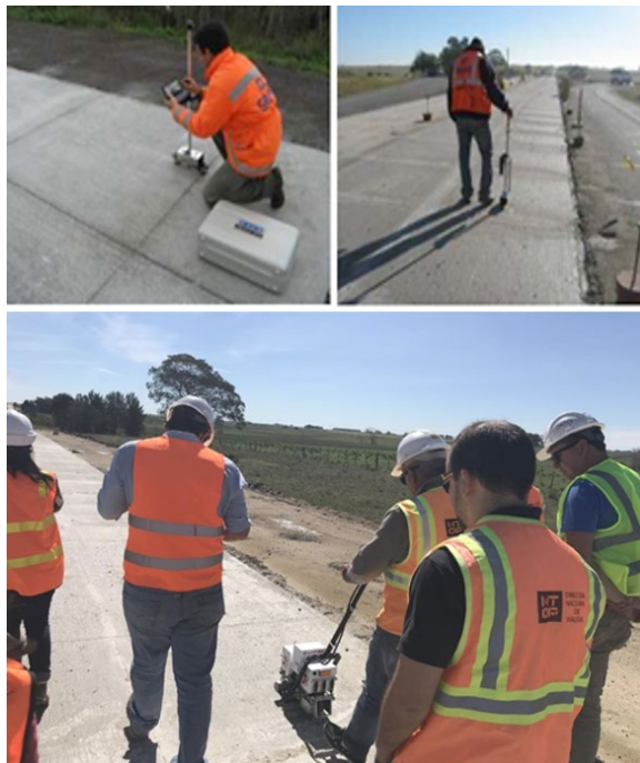
Figure 1. IRI daily check on concrete pavements with rotating inclinometer(top) and with SurPro (bottom)
