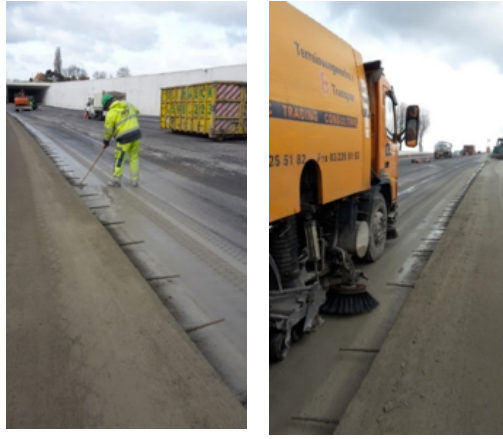
Figure 12. Cleaning of the asphalt layer next to freshly placed concrete after exposure of the aggregates at the surface
