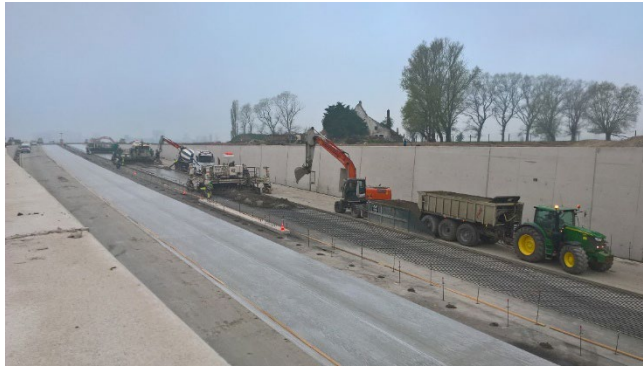
Figure 9. Evolution of the construction works: placement of the reinforcement on the asphalt layer – supply of the concrete for the underlayer in a ben– spreading of the concrete with a crane – further spreading and compaction of the concrete for the underlayer with a first slipform paver – supply of the concrete for the top layer in a mixer – spreading of the concrete with crane – further spreading and compaction with slipform paver – spreading of retarder and placing of plastic sheet over the surface
